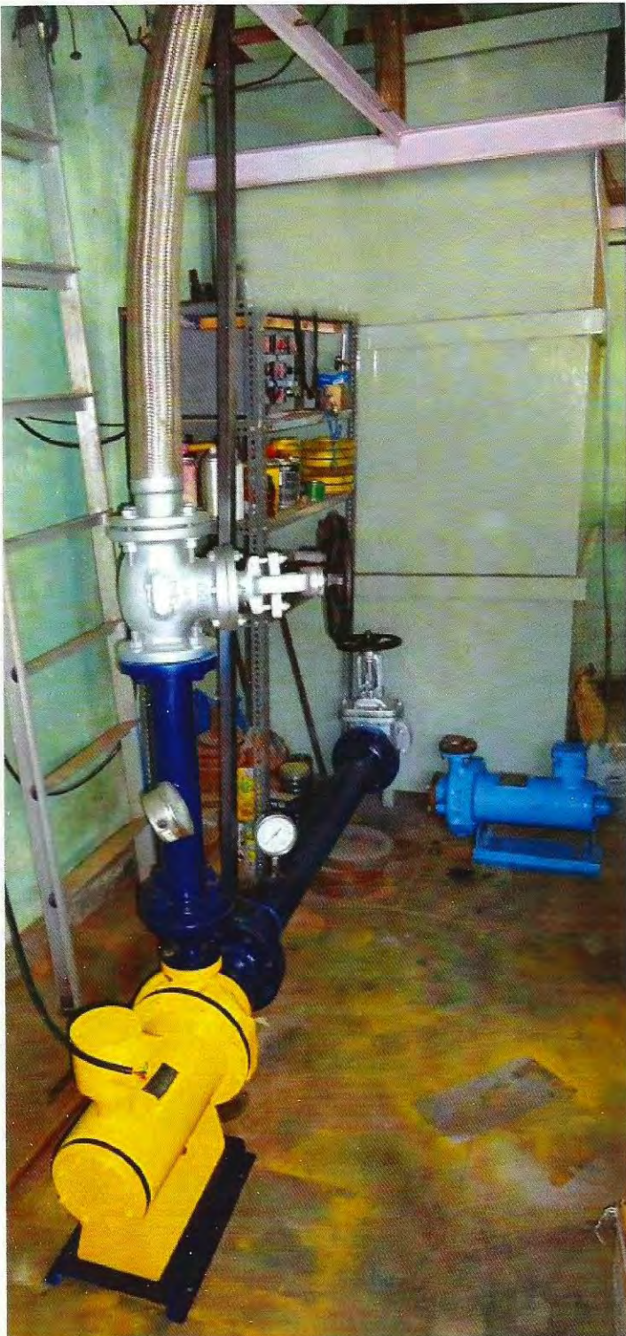
PERFORMANCE TESTING BED
